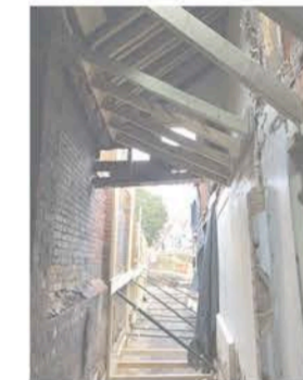
current building works showing timber frame connecting retaining wall and meeting house
