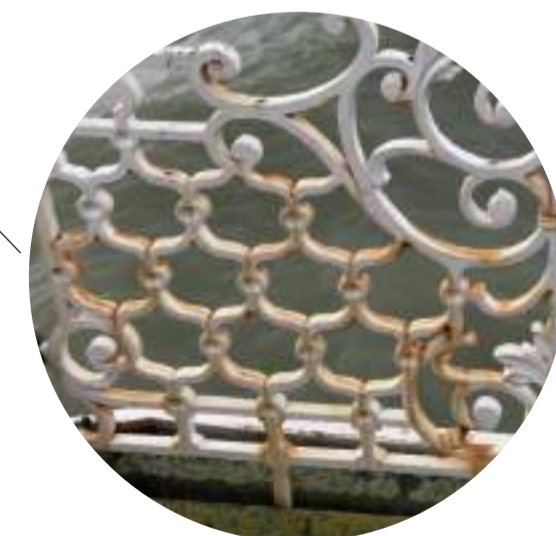
Rusted bits of iron on the pier. That can be considered as part of the design when choosing the material for my project.
