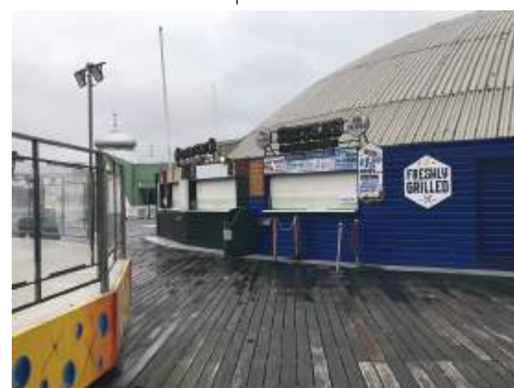
Dome to be removed - it is a mimic of the entrance's historic dome.
