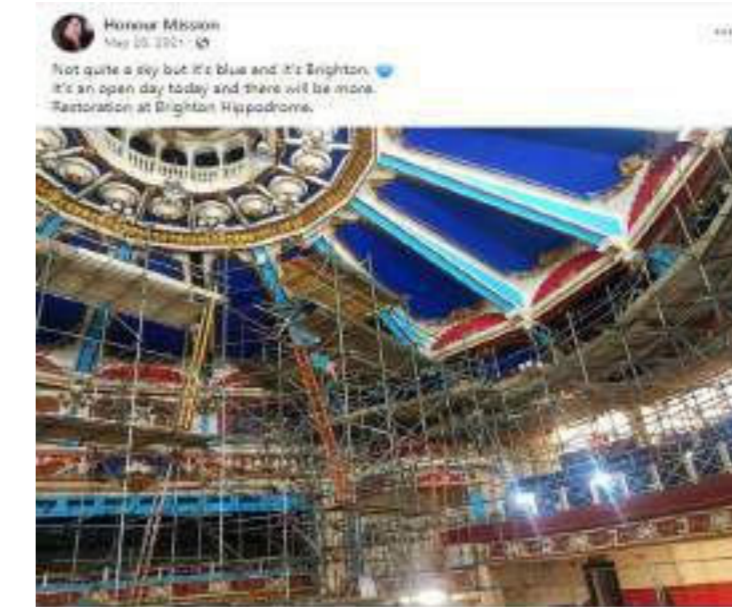
Open days at the Hippodrome for people to visit and see the repairing in progress work.
