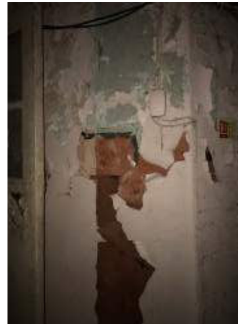
peeling of paint due to humidity and limited vapour permeability
