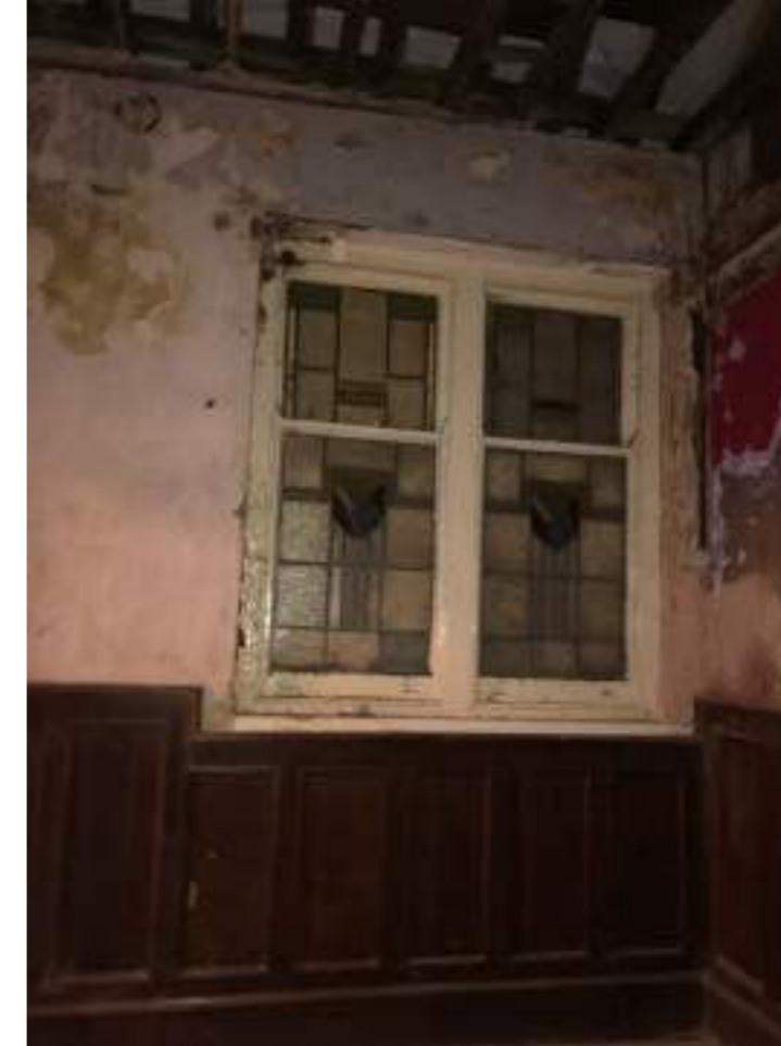
damp walls, scratched wooden panels, rusted ceiling beams
