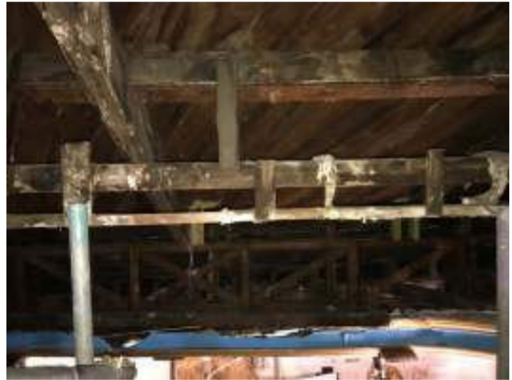
efflorescence, white powdery substances on the ceiling structure due to water flowing
