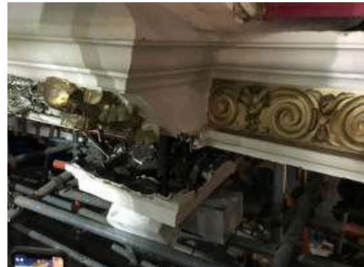
Chipping/spalling where the structure is split and separated into fragments. Bursts and uneven breaks due to uneven compression
