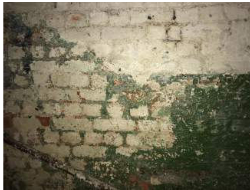
organic growth caused by being wet
