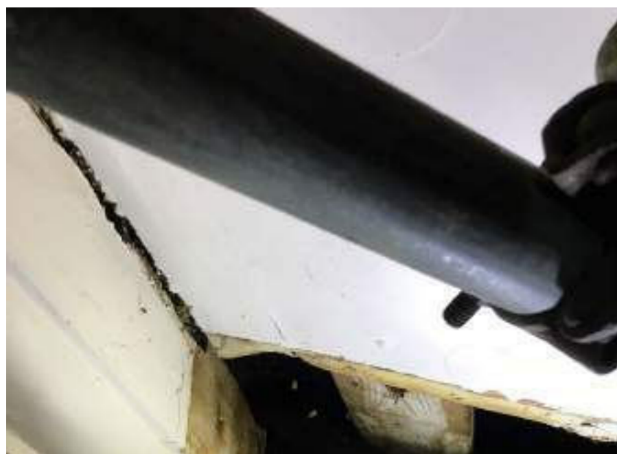
large cracks and separation between beams due to high stress exceeding resistance over time
